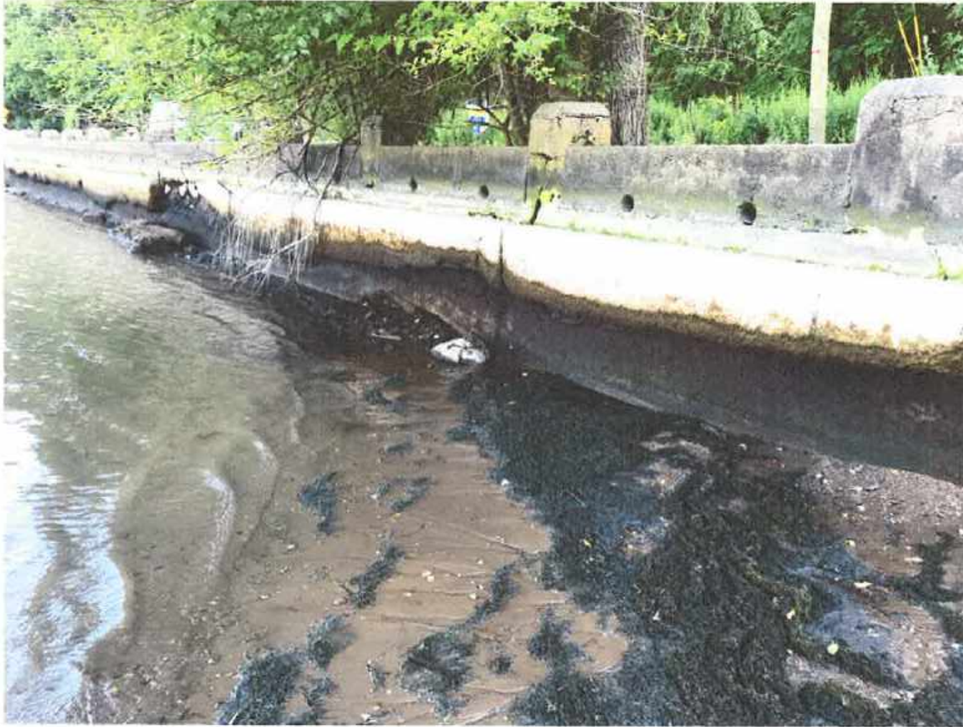
Beach Road along existing deteriorating sea wall – river side north end
