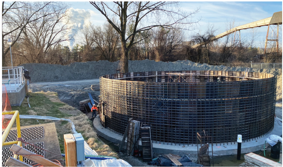
The second of two new clarifier tanks under construction at the Wastewater Treatment Plant.
